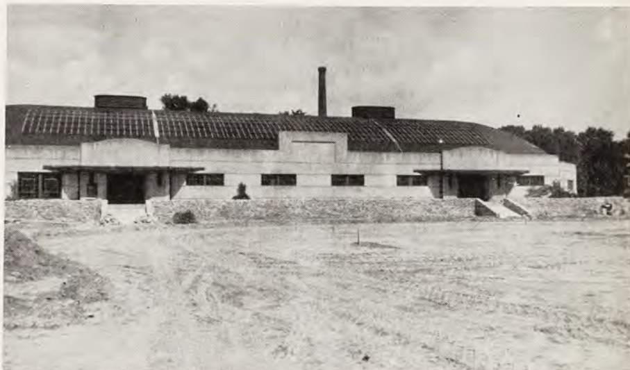
PROGRESS ON ATHLETIC FIELD. This photograph shows the late summer status of preparations for Swarthmore's new athletic center, scheduled for use in 1951-52. In the foreground is the future playing area, once the site of a dump, already levelled off for planting and construction. At the rear is the south side of the Lamb-Miller Field House.
