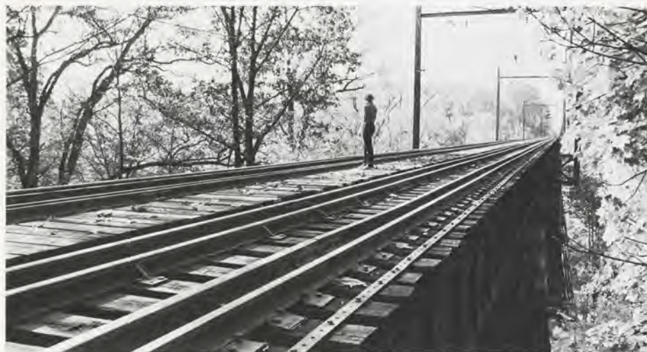
THE END OF THE LINE: The railroad trestle, scene of legendary undergraduate escapades through the decades, is currently undergoing extensive repairs. Spanning Crum Creek, the trestle links sections of track between Swarthmore and Wallingford. Trains operating on the Media Local line are now being halted at Swarthmore and passengers traveling farther west must continue by bus. Trestle repairs should be completed by October.
