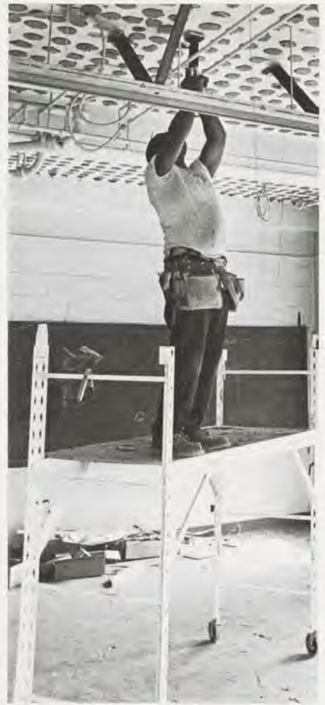
A workman installs a new ceiling as part of the modernization of Martin laboratories.
